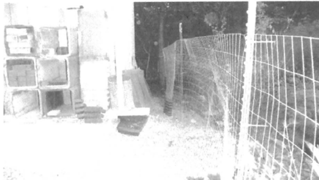
Image 2. West wall of the structure is about two feet from the adjacent lot line
